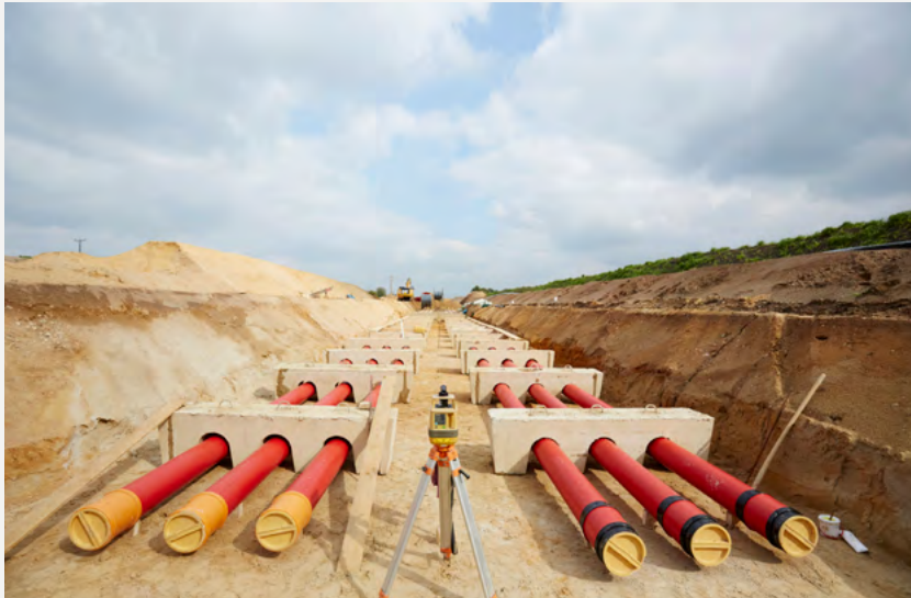
Rhein-Main-Link project. Image by Amprion
